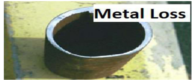
Figure 8. Example of Metal Loss
