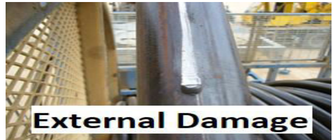
Figure 9. Example of External Damage
