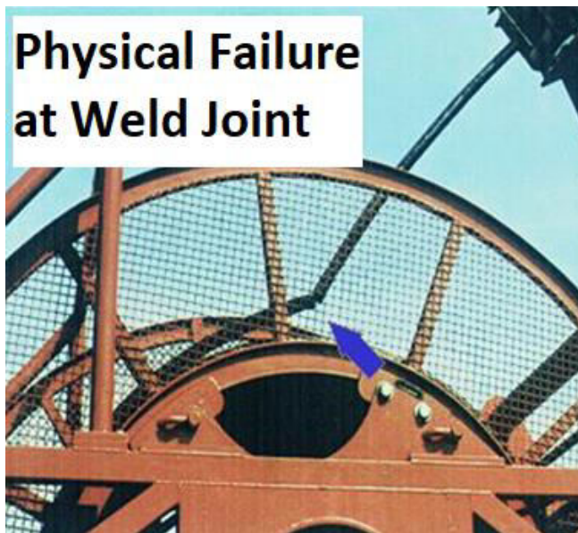
Figure 6. Failure due to Physical Failure at Weld Joint
